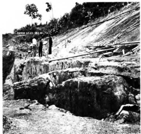
Fig 4: Subsidence at EL 263 m as on Nov'2006 (view to west)
